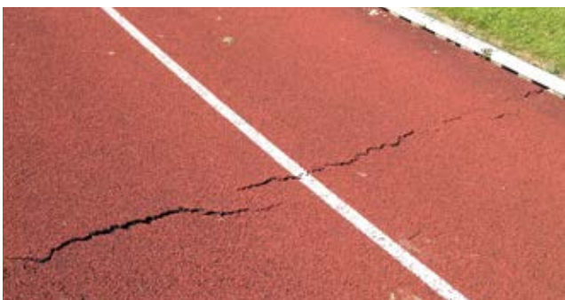
Clearly apparent cracks
