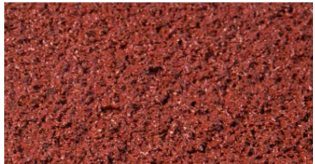
Good example: Clean surface
